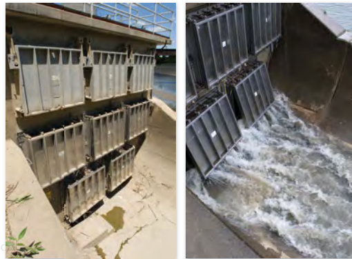
Lick Run CSO in South Fairmount under dry and wet conditions
