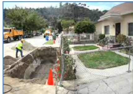
Constructing green infrastructure features in locations with poor sidewalks improves water quality and pedestrian facilities. (City of Los Angeles 2010, www.lastormwater.org )
