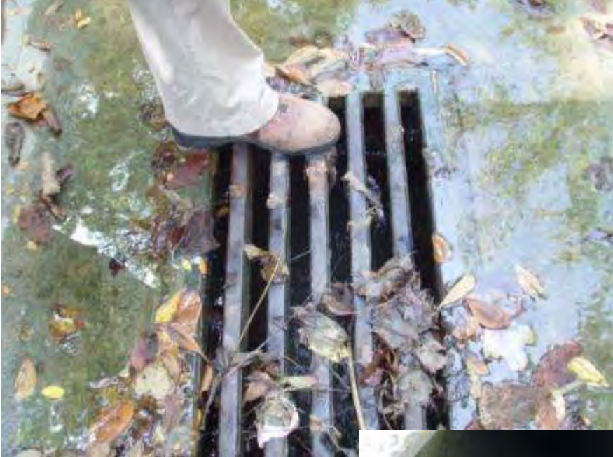
Invert Grates Connect Channel to Interceptor
